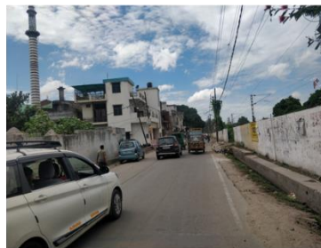
P1 Road Condition
