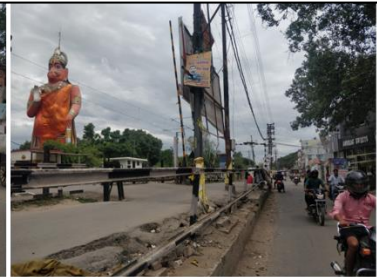
P1 Road Condition
